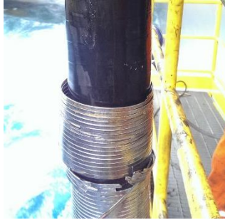
Damaged stainless steel wrap
